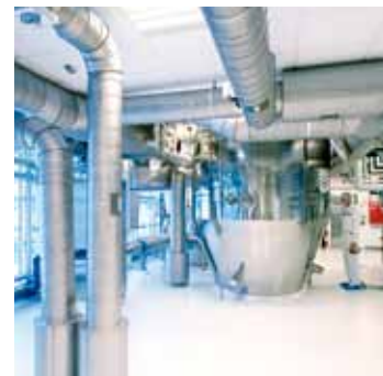
GEA Niro PHARMA SD™ type PSD-4 chamber and HVAC ducts.
